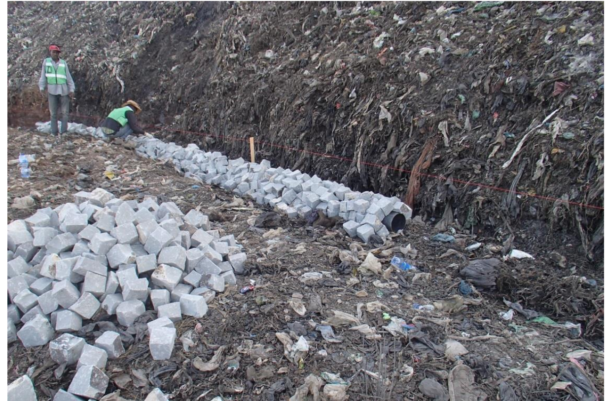
Installation of Leachate Collection Pipe at Koshe (Rappi) Landfill Site (2018) (Source: Materials of ACCP Study Tour)
