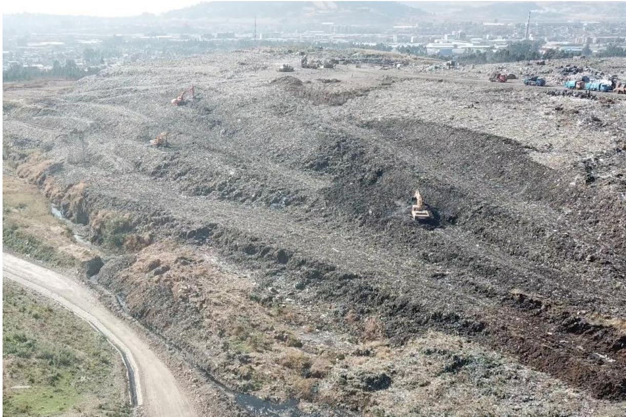
Improvement Works at Koshe (Rappi) Landfill Site (2018) (Source: Materials of ACCP Study Tour)
